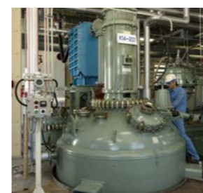
Reactor: 8000 L Glass-lined
